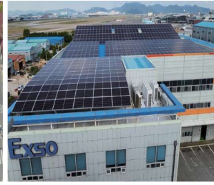
Distribution Complex with Curved Roof (200 kW)
