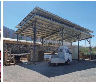
Parking Lot Solar Power Plant (100 kW)
