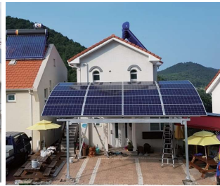
Residential Solar System (Parking Lot Type)
